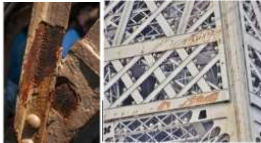
Figure (11): corrosion in the metallic structure of Eiffel Tower
