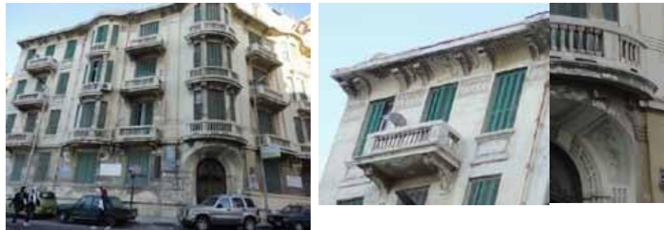
Fig. 10 : Ornamental details of an Eclectic Style residential building façade; the main entrance at the corner with classic panels and decorative foliage, balcony balustrades of repetitive ionic columns, brackets with volutes supporting balconies, a frieze surrounding the top of the building and another at the middle with a bas relief geometric pattern. (Azaritah District)
